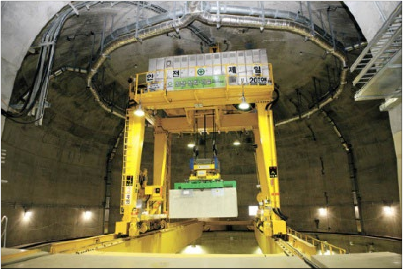
Figure 20 - Silo loading with gantry crane
